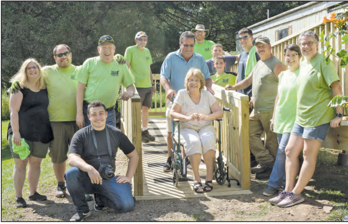
Impact Project volunteers from cvFree Church stand with Norwich homeowner Patricia Scott after building a new handicap accessible ramp as part of the organization’s 127th project. (Submitted photo)
